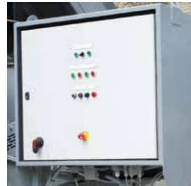
H12 Feeder Control Panel
